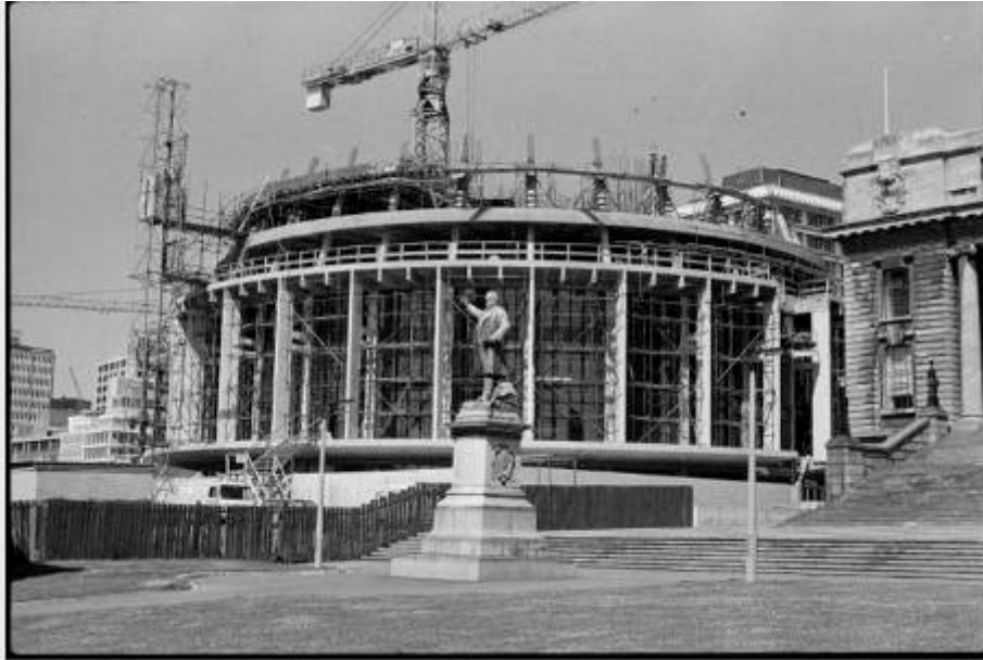
The Beehive under construction, Wellington. Negatives of the Evening Post newspaper. Ref: 1/4-022262-F. Alexander Turnbull Library, Wellington, New Zealand. http://natlib.govt.nz/records/23209583
