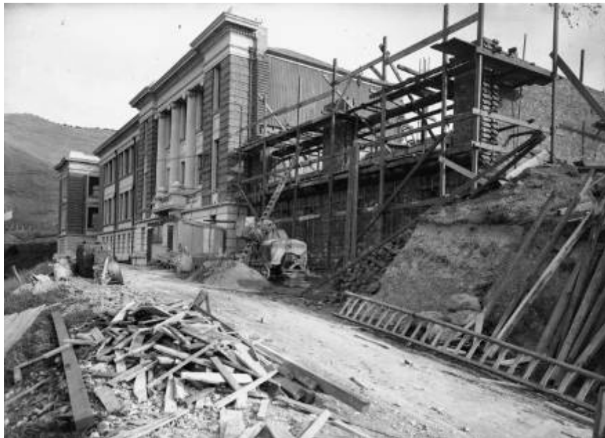
Wellington East Girls College west wing under construction, 1930. Negatives of the Evening Post newspaper. Ref: EP-1314-1/2-G. Alexander Turnbull Library, Wellington, New Zealand.
