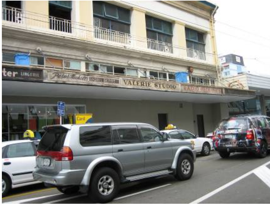
Deka Building circa 2006 – veranda facing removed to show earlier shop signage (probably from 1928 – 1951) – these appear to have been removed recently (possibly in 2010 – see SR210946 ‘Verandah panels missing’). Image WCC ref img_0692.
