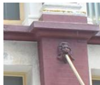
Façade details to Cuba Street. Lion or 'green man' decorative bracket at verandah support and a scroll at column capitals.
