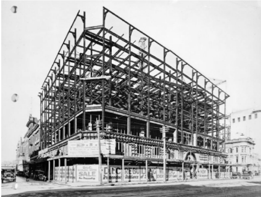
1928 DIC department store under construction, steel structure . Image: FG Barker, WCC Archives 00138_0_11044
